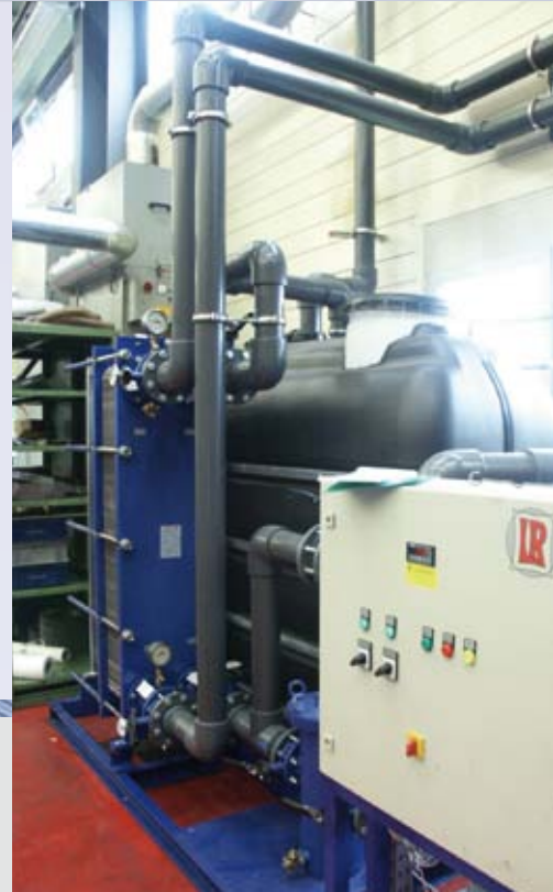
Cooling of lubricating oil for extruding presses.
