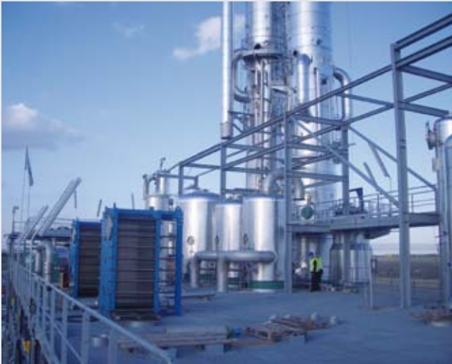
Condensation of bioethanol.
