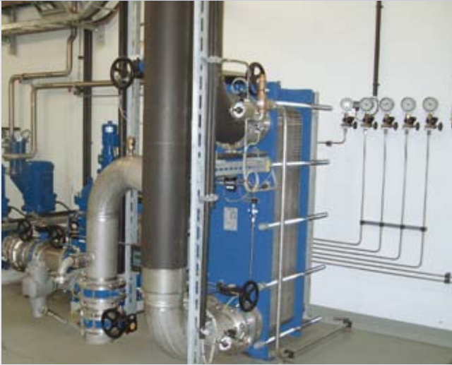
Hydraulic oil cooling in power plant.
